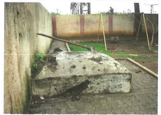
Remains of Electric Tower
