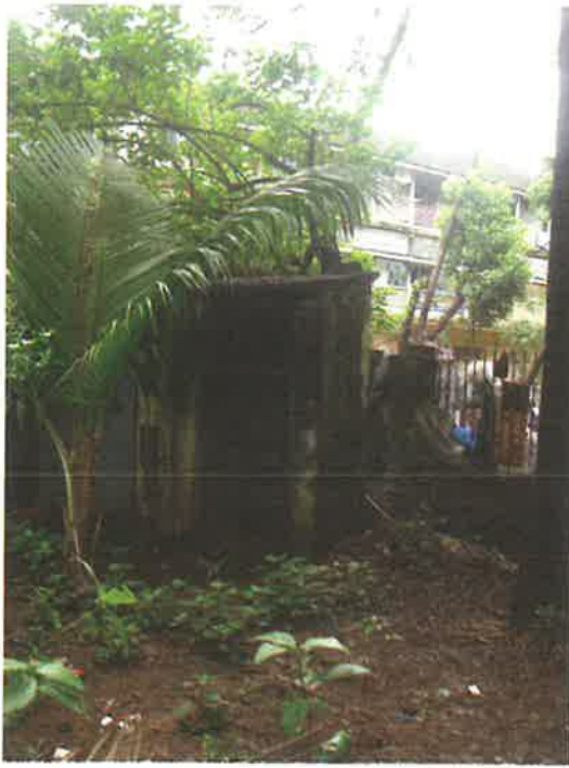
Electric room (2.8x1.2m) at Southeast corner of garden
